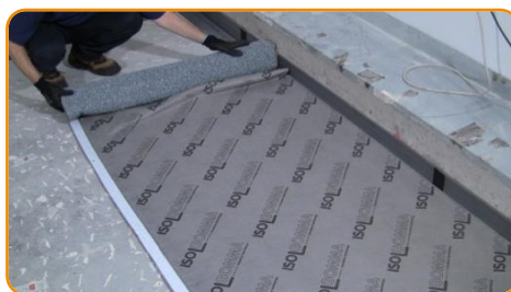
Lay down the insulation layer on the floor surface with the rubber granules turned on the bottom floor side.
