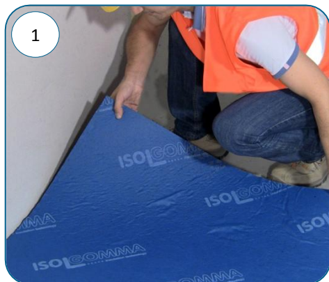
1 Lay the Matrack mats on the pit, without leaving gaps between adjacent mats or along the edges
