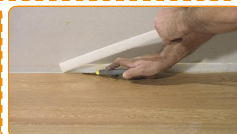
When the flooring application is completed, cut the exceeding part of the
